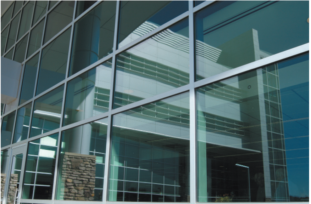
As windows become larger-- and the demand for natural light grows-- glass plays an ever-increasing role in the overall appearance of commercial buildings.
